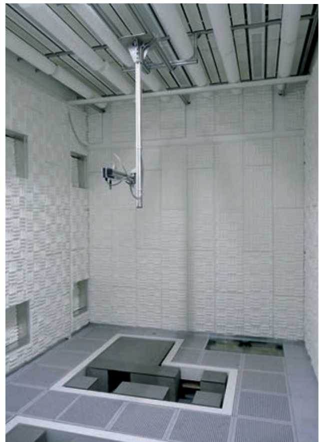
Experimentation room with 4.2 m clear room height and acoustic insulation materials (supplied and installed by Bilz).
